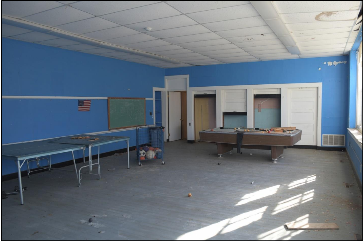
Figure 24: North classroom, facing southwest
