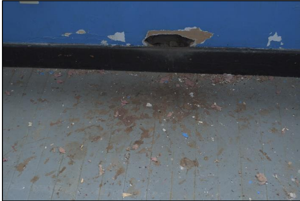
Figure 74: Rodent hole below north classroom windows
