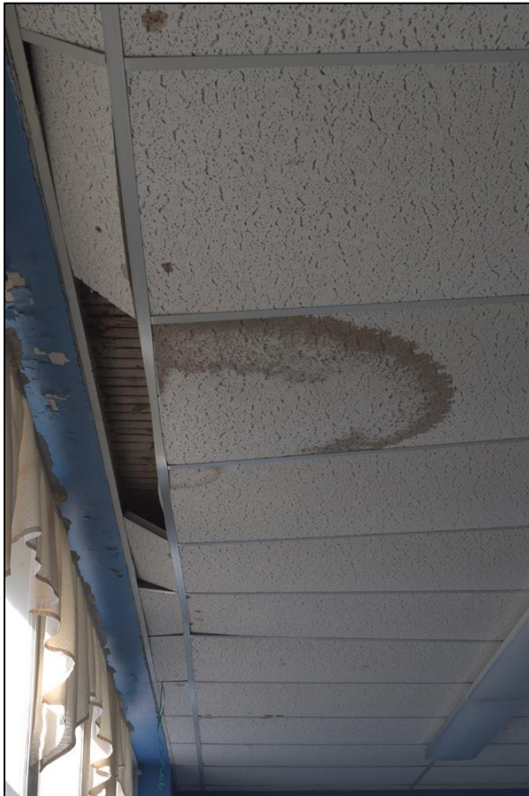
Figure 76: Water damage to ceiling above north classroom windows
