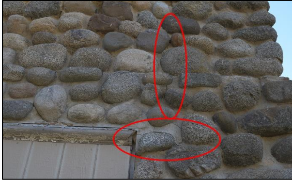
Figure 63: Cracks in cobblestone at east elevation
