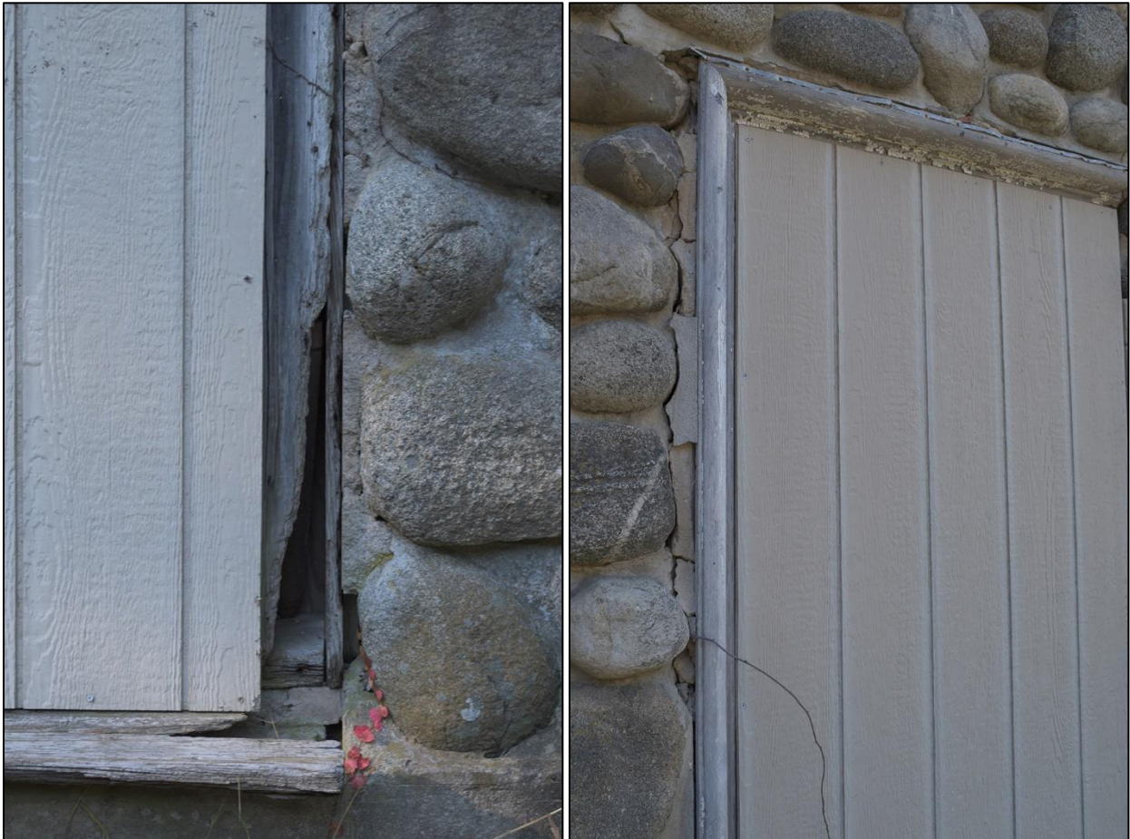
Figures 66 & 67: Details of lower level windows, showing damage to window casings (note large masonry crack at right image)
