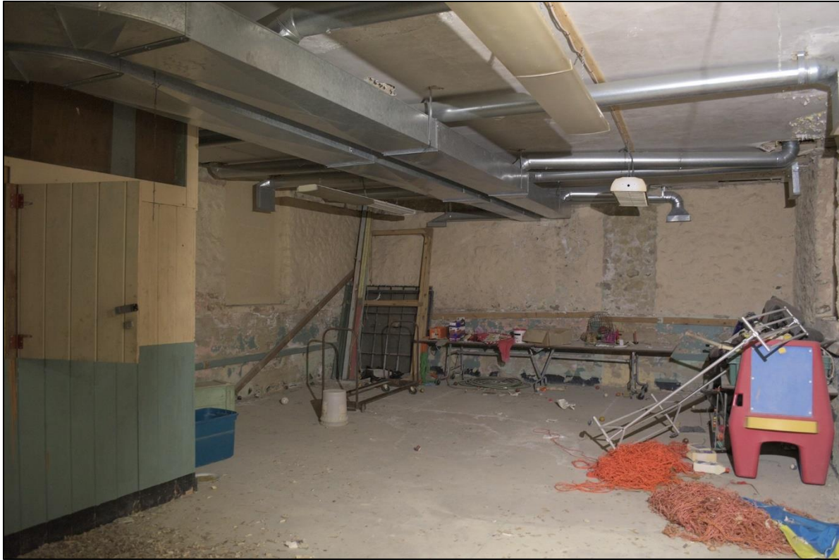
Figure 40: North storage room, facing northwest with ca. 1948 storage room/closet in foreground at left
