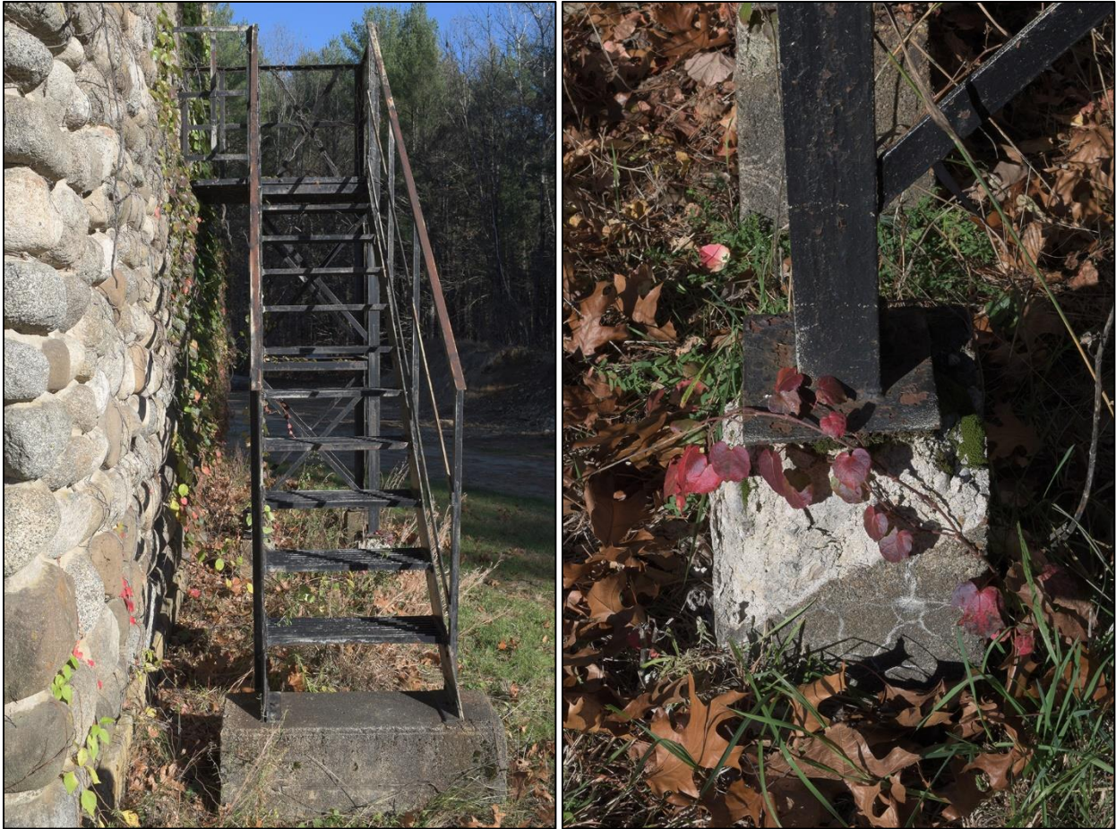
Figures 71 & 72: South fire escape stair configuration (left) and damage to concrete base (right)
