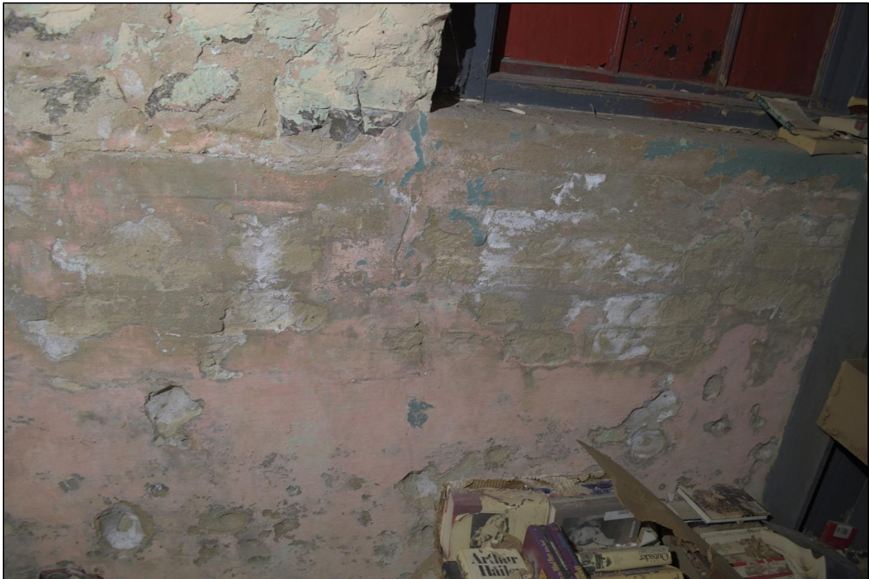
Figure 78: Efflorescence at west wall of north classroom (inside of built-in closet)
