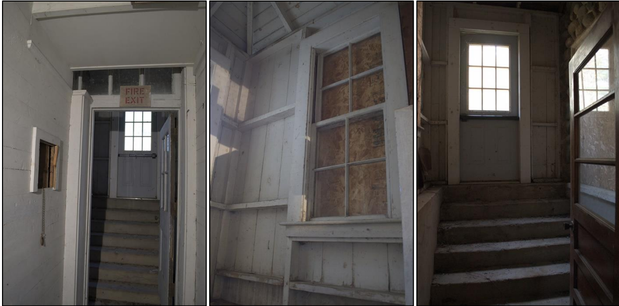
Figures 46, 47, & 48: North basement exit, photographed from vestibule showing alteration at west door jamb (left), window at north basement exit (center), and south basement exit (right)
