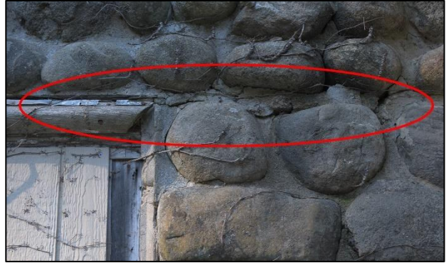
Figure 64: Cracks in cobblestone at west facade
