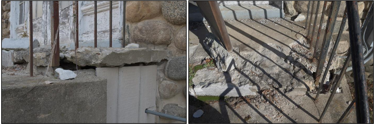
Figures 69 & 70: Damage to landing at south side of steps from the side (left) and above (right)
