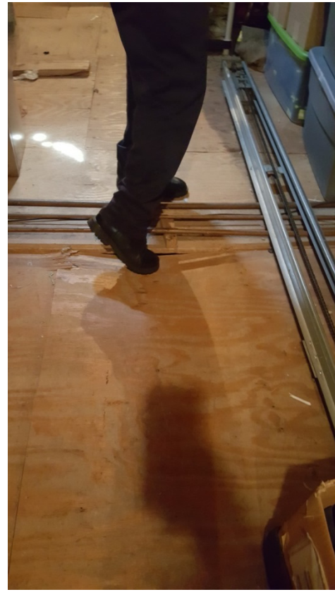
Figure 34 Unsafe floor in attic over admin area
