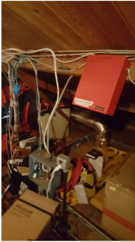
Figure 33 Storage around electrical in attic space over admin area
