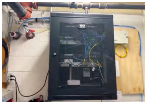
New Network Closet
