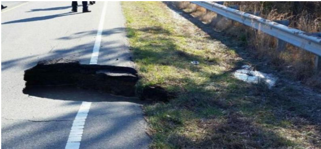
Sink hole picture
